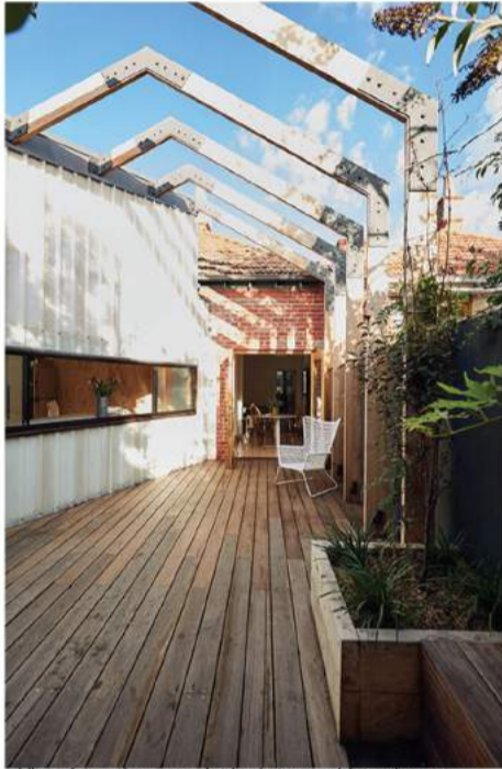
View from the new decked area, with a view to both the existing house, and the new addition on the left. Exposed structure will become inhabited by vegetation as the landscape adapts to the addition.
