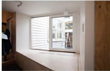
Library link, looking out: Seat to enjoy reading, with a direct view into the courtyard, existing weatherboards visible
